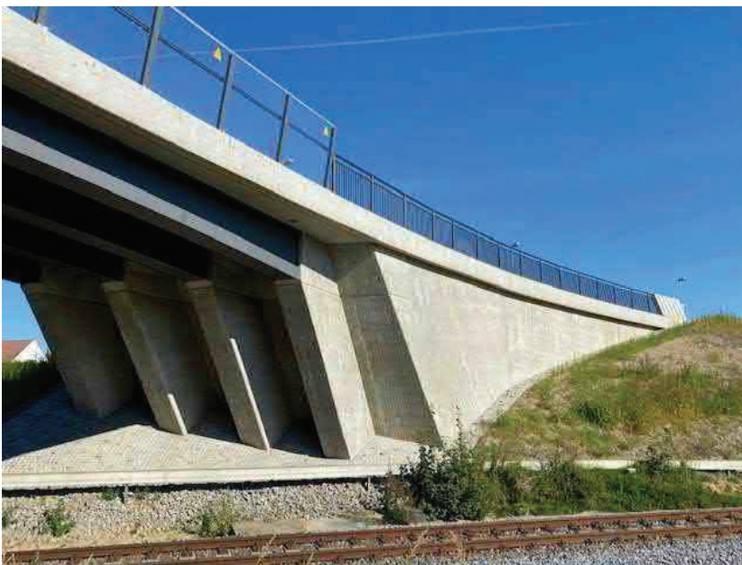
Many bridges such as this road bridge crossing a railroad line at Großbarthau in eastern Germany feature super-elevated curves and changing gradients.
