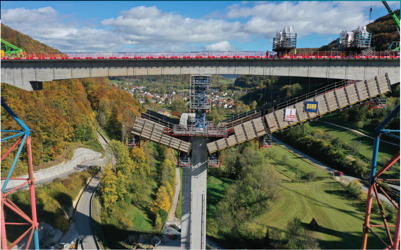
The semi-integral bridges are supported by slim, Y-shaped piers with flat-angle struts that were concreted and seamlessly connected to the beams at the end of the construction process.
