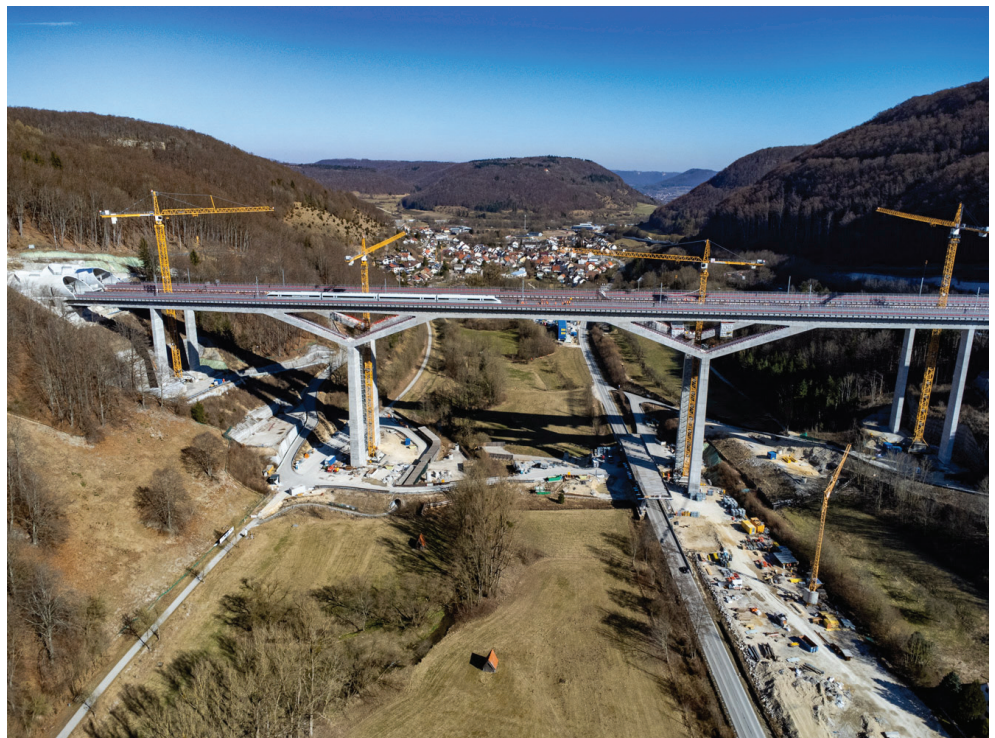
The dual bridges across the Fils Valley in southern Germany are part of the Stuttgart to Ulm segment of the European high-speed line linking Paris, Munich, Vienna, Bratislava and Budapest.
